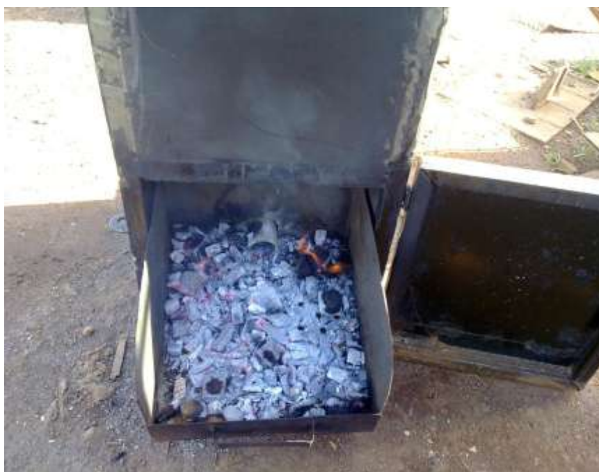
Plate 3. The boiler showing incomplete combustion of biomass
