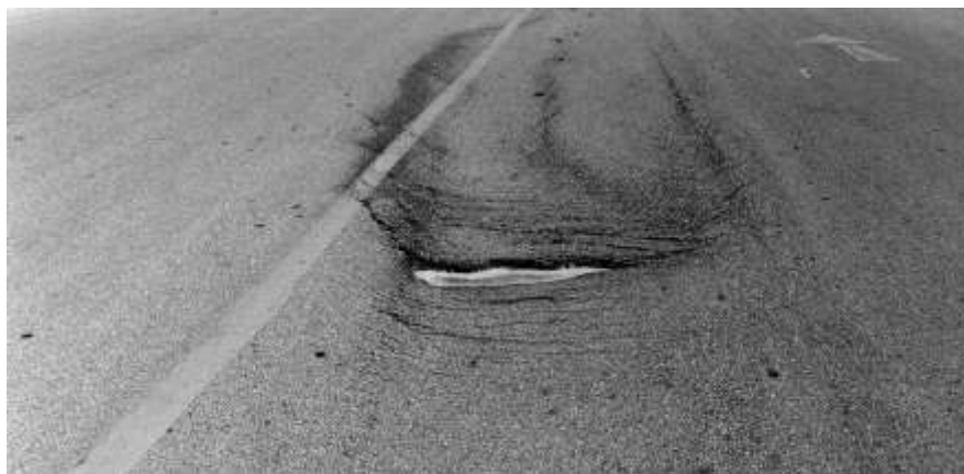
Figure 1.1: Slippage Crack ( http://www.surface-engineering.net )
