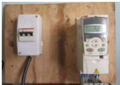
Fig 2.2 VFD (Variable Frequency Drive)
