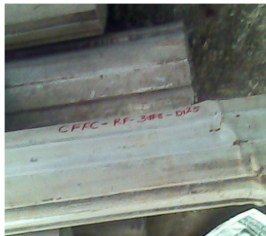
4(d) Failure of column CFSFC L/D 20 at bottom with 3/#8
