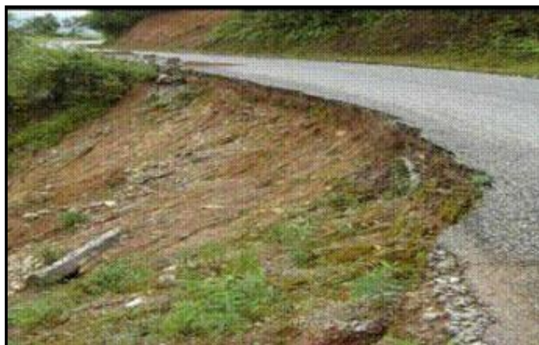
Figure 10: Pavement Failure due to Slope Instability, adapted from Hearn et al. [22].
