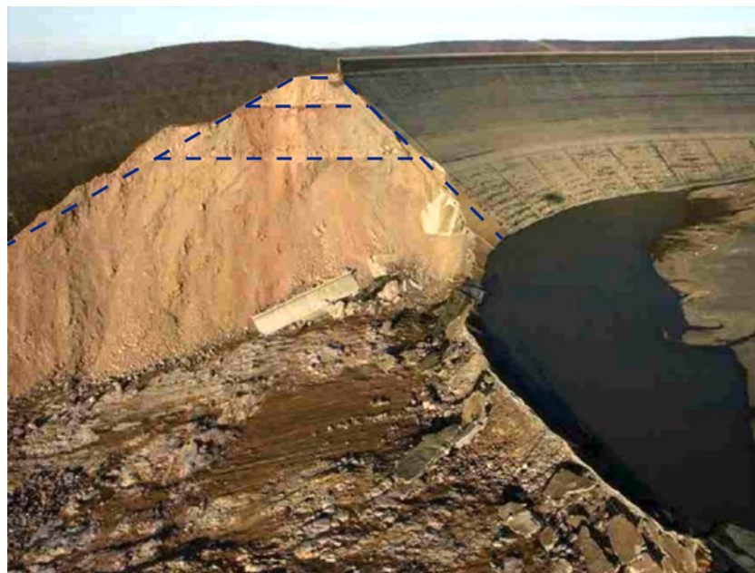
Figure 3 Photo of dam materials in the breach side slope, W. M. Wu.
