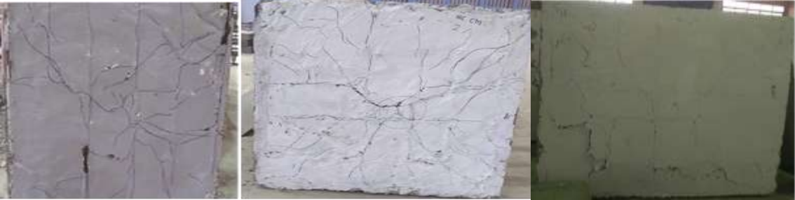
Fig 8: crack pattern of the tested slabs for group (3).
