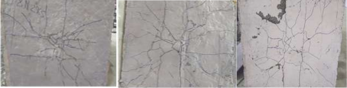
Fig 7: crack pattern of the tested slabs for group (2).
