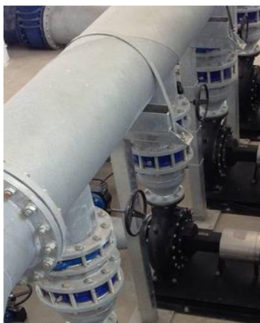
Figure 6. Water pressure reduction station in the Alexandria city, Romania
