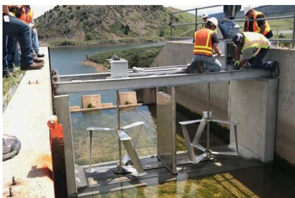
Figure 4. Placement hydrokinetic turbines in a irrigation canal
