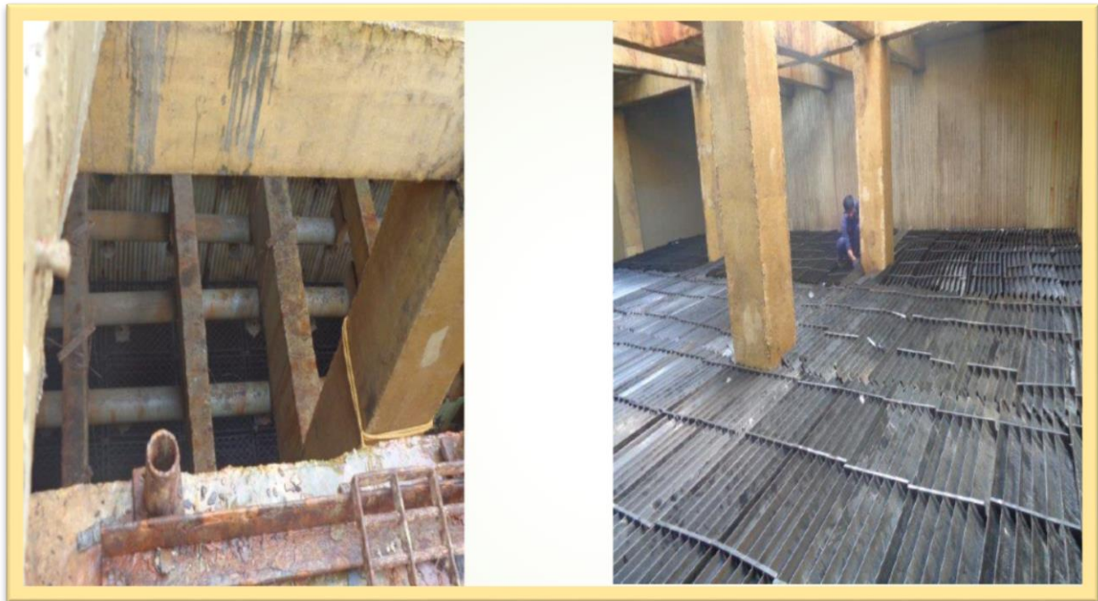
Picture 4 : DISTRIBUTION PIPES (left photo) ON WHICH DRIFT ELEMATOR MOUNTED(Right photo)
