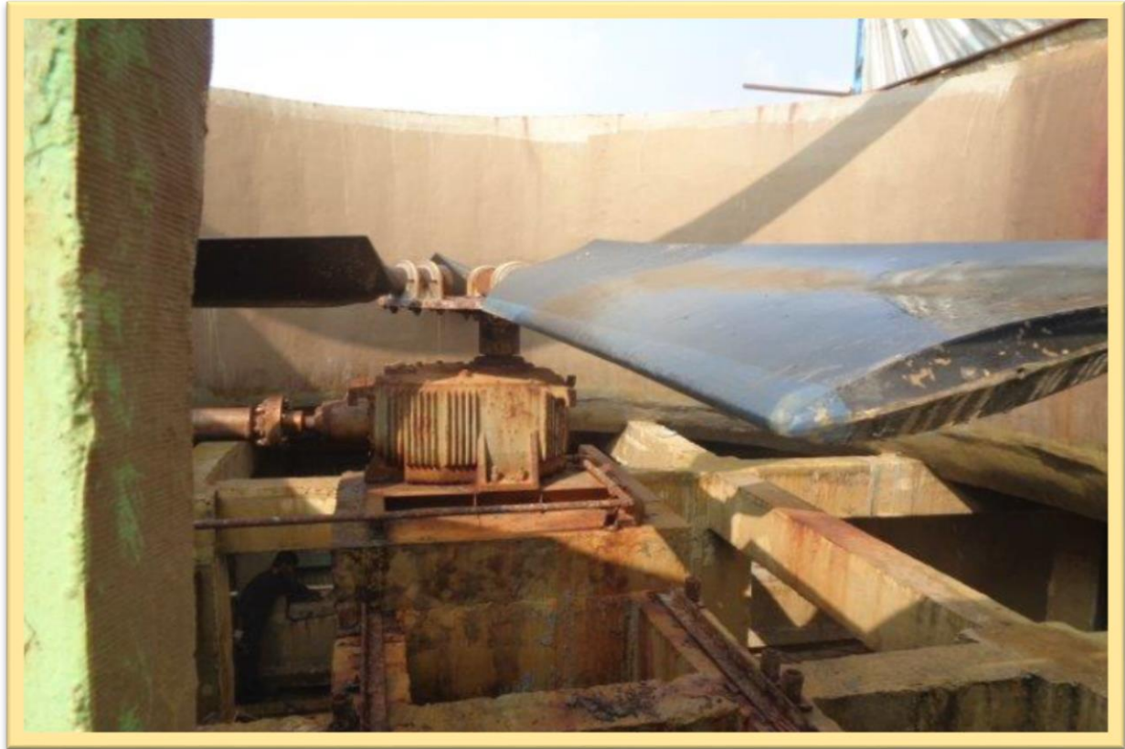
Picture 6 : Gear Box with 4 no Blades of Induced Fan Assembly
