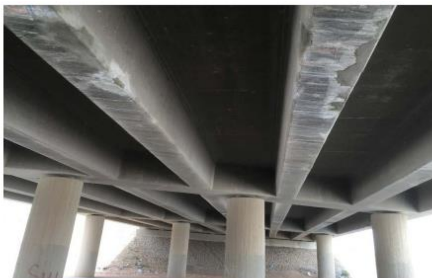
Figure 2 Side view of the Al-Fahs bridge and view of the lower deck, respectively (Riyadh, KSA).
