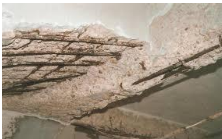
Figure 3. Show steel reinforcement rust and concrete cracks due to rust
