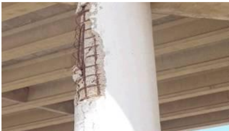
Figure 4. Show cracks in the columns, A. Because of the forces acting; B. Because of the technology of implementation.
