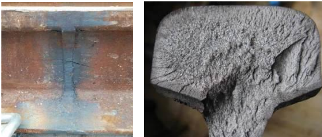
Fig 2 Defects in rail butt welded joints
