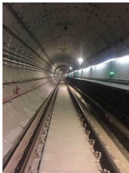
Fig 8 Fully lock the rail at the design fixed temperature of rail stress release
