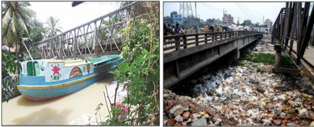
Figure: Picture of poor bridge side
