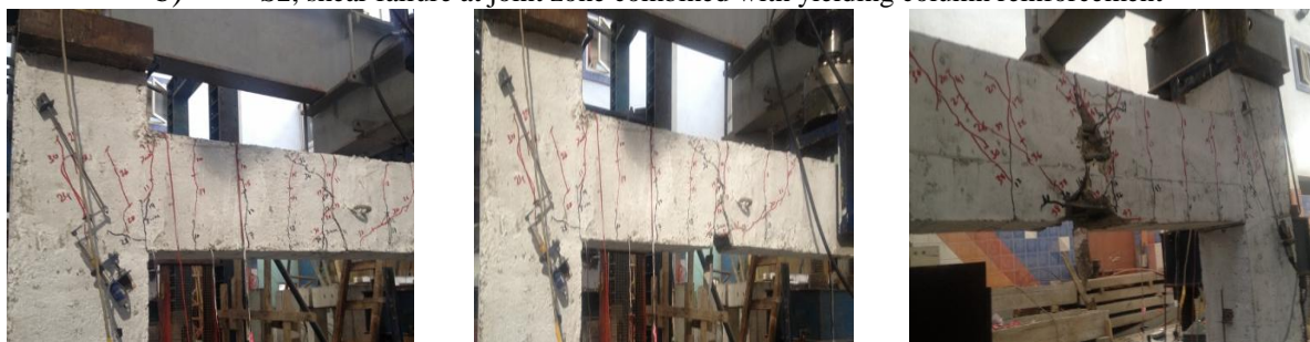
c) S3, brittle shear failure of concrete at end of encased steel section in beam zone
