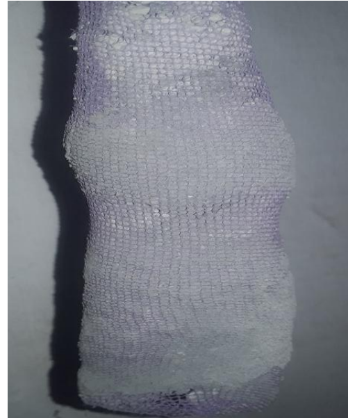
Figure 4: Bulging of Encased Stone Column
