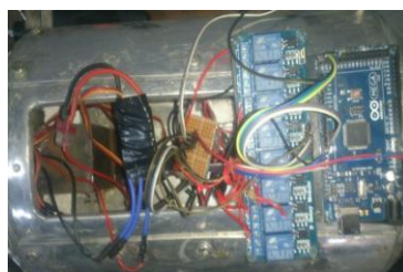
Fig. 14 Setup of control panel
