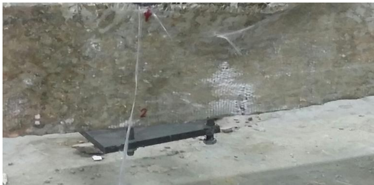
Figure 12 Rupture of GFRP sheet
