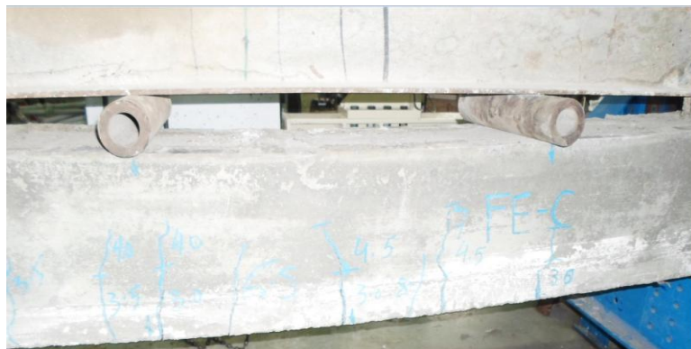
Figure 8 Strengthened beam (FE-C-B) cracks Pattern
