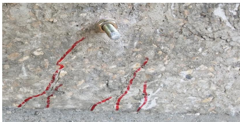
Figure 14 Cracks pattern for strengthened beams after removal of GFRP sheets G2-B
