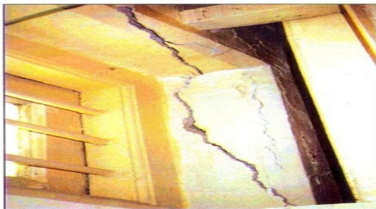
Figure 1.4 Crack in concrete due to corrosion of steel
