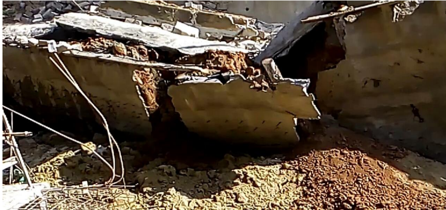
Fig 5. The scene of the collapsed accident (East corner side)
