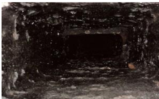
Fig. 4 Creosote deposit on chimney
