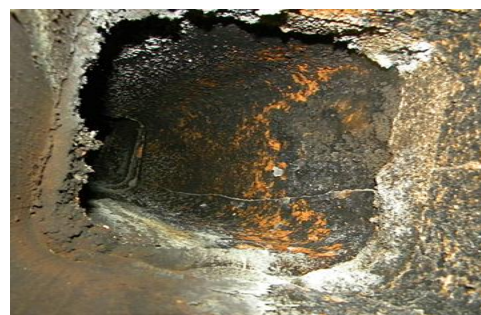
Fig.5 Soot deposits on chimney
