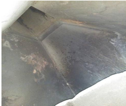
Fig. 14: Chimney before cleaning
