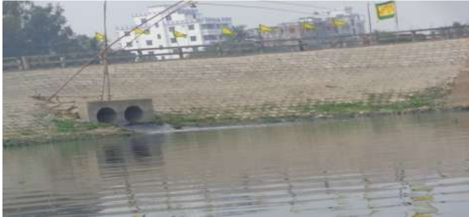
Figure 8: Storm sewers Outfalls of Turag River
