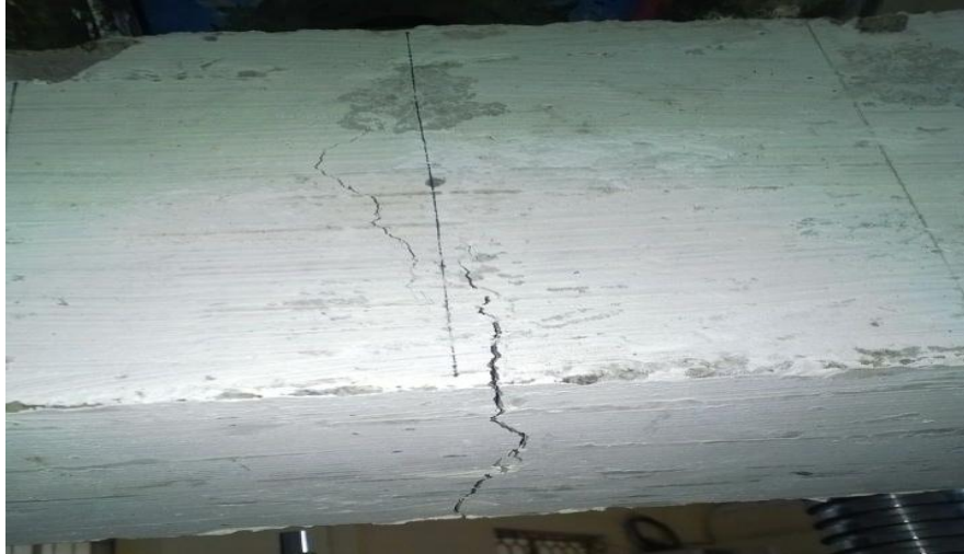
Figure 12: Failure of Plain Concrete Beam (1)
