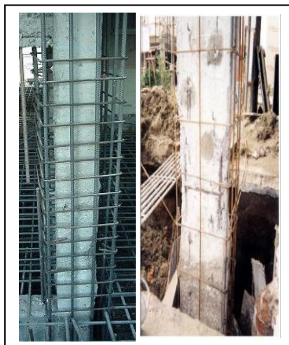
Fig 1. Picture showing column jacketing
