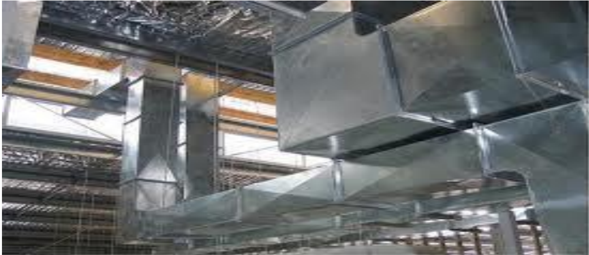
Figure 2. Site view of Rectangular duct with 90° bends
