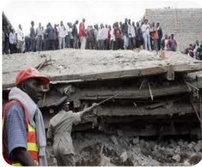
Fig 1: collapsed four storeys in kisumu, Kenya.
