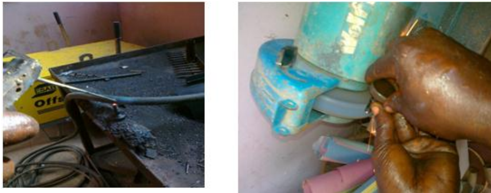
Fig. 6: Welding and grinding of the deformed lock nut tip
