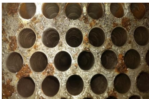
Figure 1: Before scale removal
