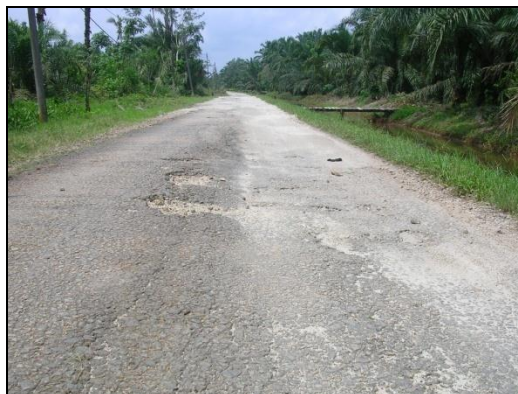
Figure 1: Impact from road drainage structure failure for rural road in Parit Raja
