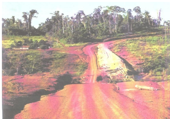
Plate 4: A collapsed road in Ikoe Ikot Nkong of Ini Local Government Area – An adverse consequence of sand dredging in the area.
