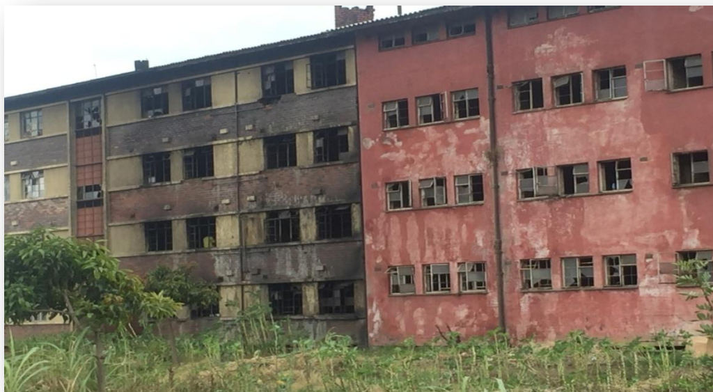
Figure 4.3 Deplorable state of Block 1 -Sidojiwe hostel.
