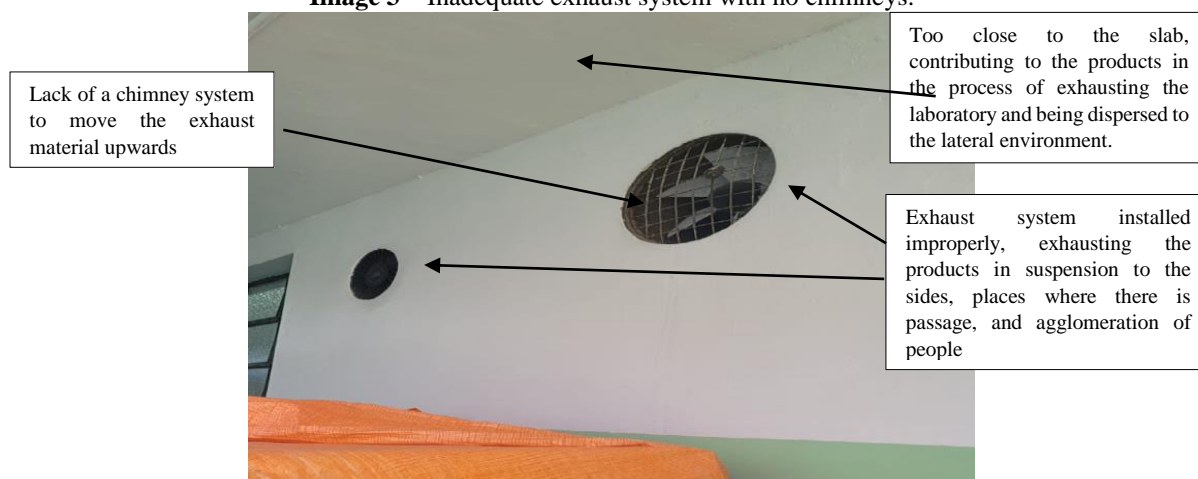
Image 3 – Inadequate exhaust system with no chimneys.
