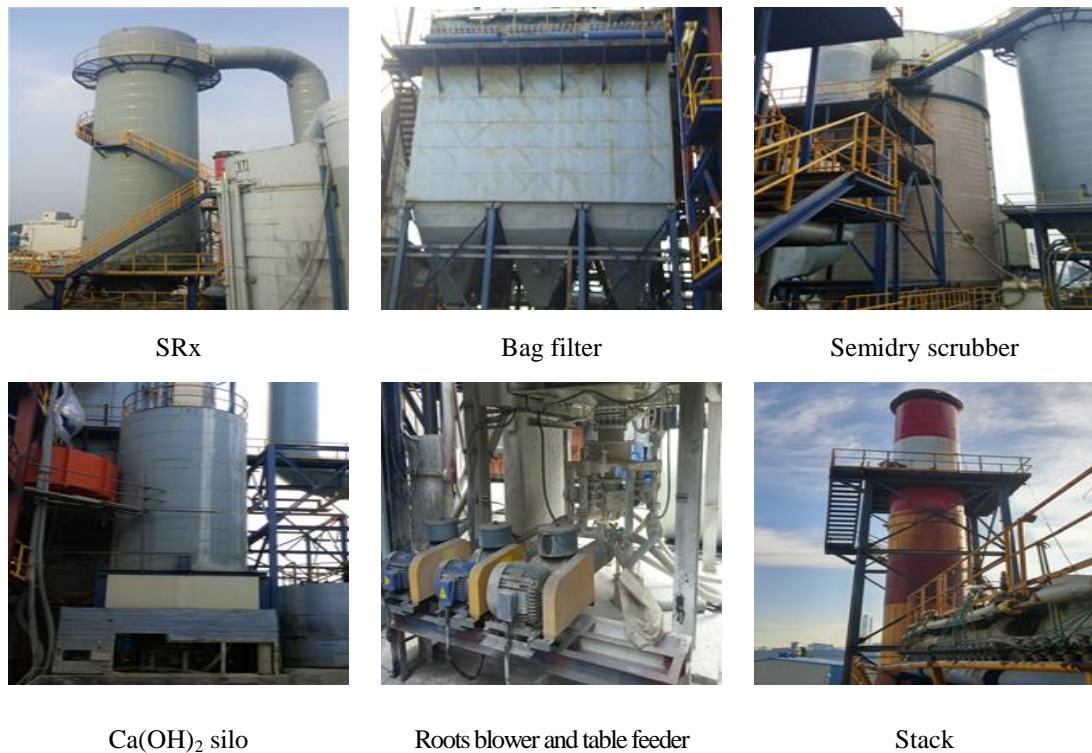
Fig. 4. Functional units of the air pollution prevention facility of the municipal waste incinerator
