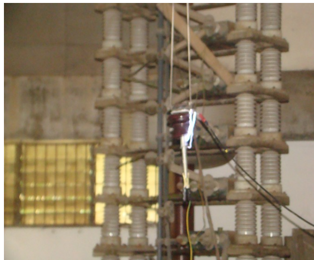
FIG 8: Contamination of Insulator with Co and the Flash over voltage Spark.
