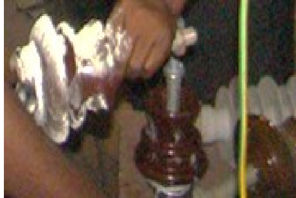
Fig 7: Contamination of Insulator with Cement
