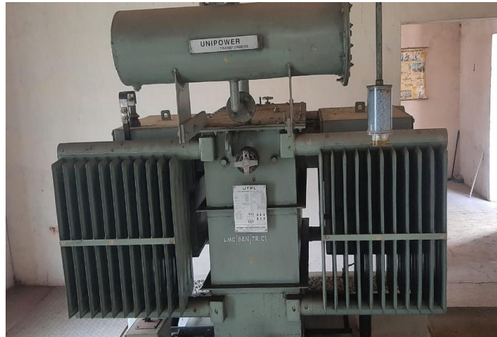
Fig.3: 400 KVA, 11kV/433V distribution transformer
