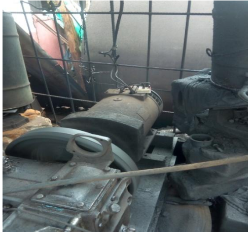
Plate 1 – Water cool, diesel engine operated alternator.
