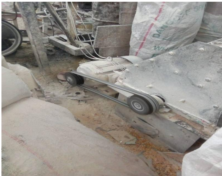
Plate 4: An induction motor (electrical load) fed with 415V, 3-phase lives and driving a grinding mill (mechanical load). Courtesy: Eke-Awka grinding mill lines, Anambra State.
