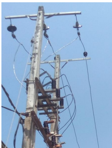
Plate 3 – Transmission line, feeding a distribution transformer, near K.A.C lodge Ifite Awka.
