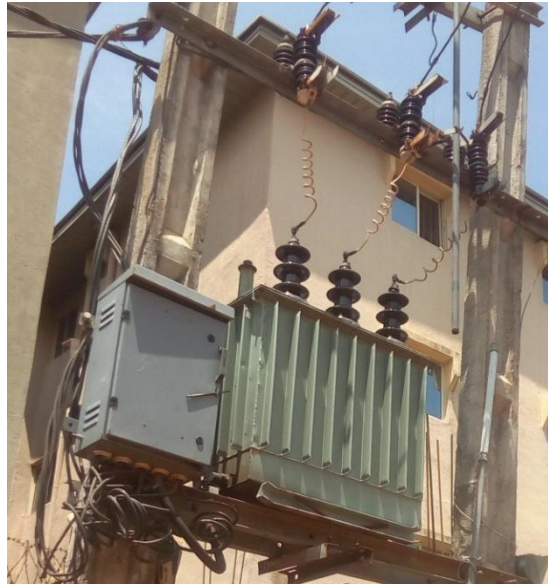
Plate 2 – Power distribution transformer, near K.A.C Lodge Ifite Awka
