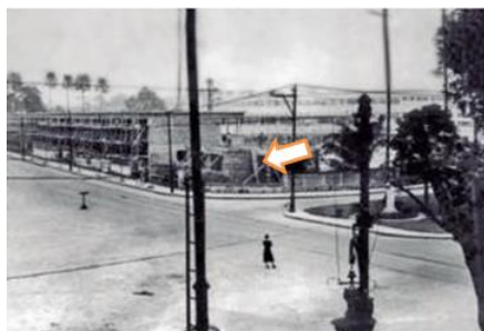
Figure 3: External View Of Blocks D And F Under Construction On General Canabarro Street 14 .
