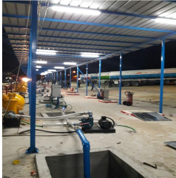
Figure (2) Petrol Vehicles from the Egyptian Side during discharge at the Rafah petroleum crossing. Source: The researchers
