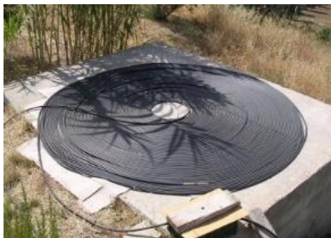
Figure 7: Exposed coiled hose solar collector (Hare, 2014).
